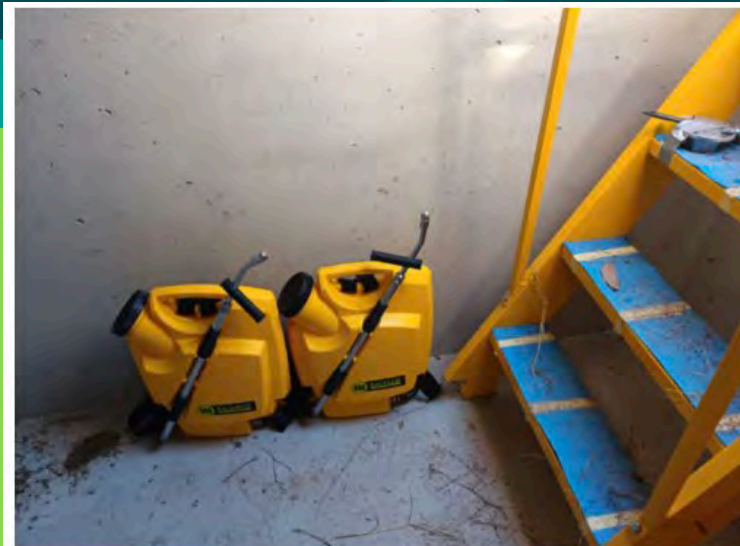
Firefighting knapsacks in a bunker ready for use.
