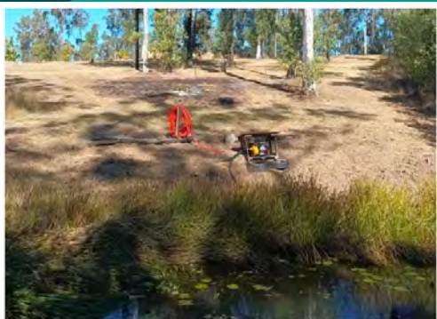
1.4 Davey double impeller pump/ hose installed.
