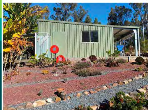
Fire reel installed
