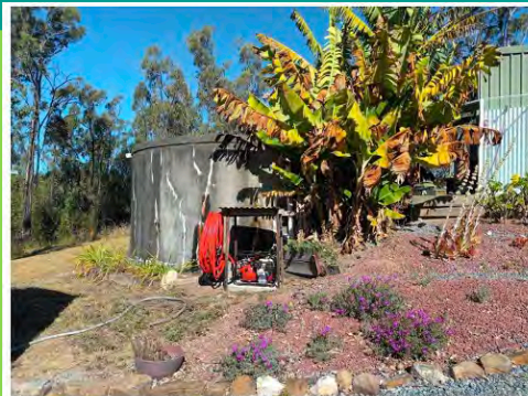
1.4 Davey Single Impeller pump installed.
