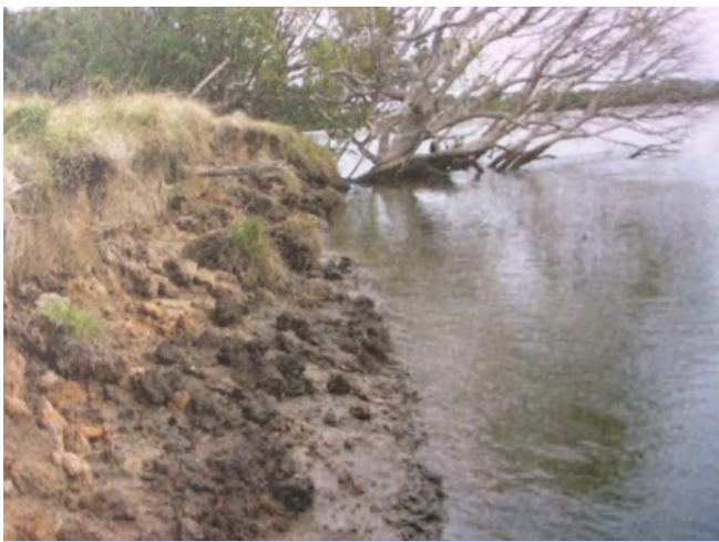
Problem: river bank eroded with resultant loss of mangroves and fish habitat
